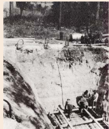
GEORGETOWN, SC – Excavation for sewage pumping station. Also begun in the 1950s, this site was one of five planned for the sewer system of the "Maryville Section" which was eventually annexed to the City of Georgetown in 1957. W.K. Dickson's project description made special mention of "...the use of the Well Point System to control ground water during construction."
